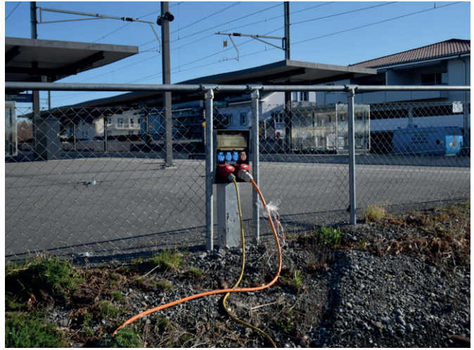
Power distribution box at Oberriet railway station
