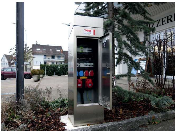
QUADRO power column
